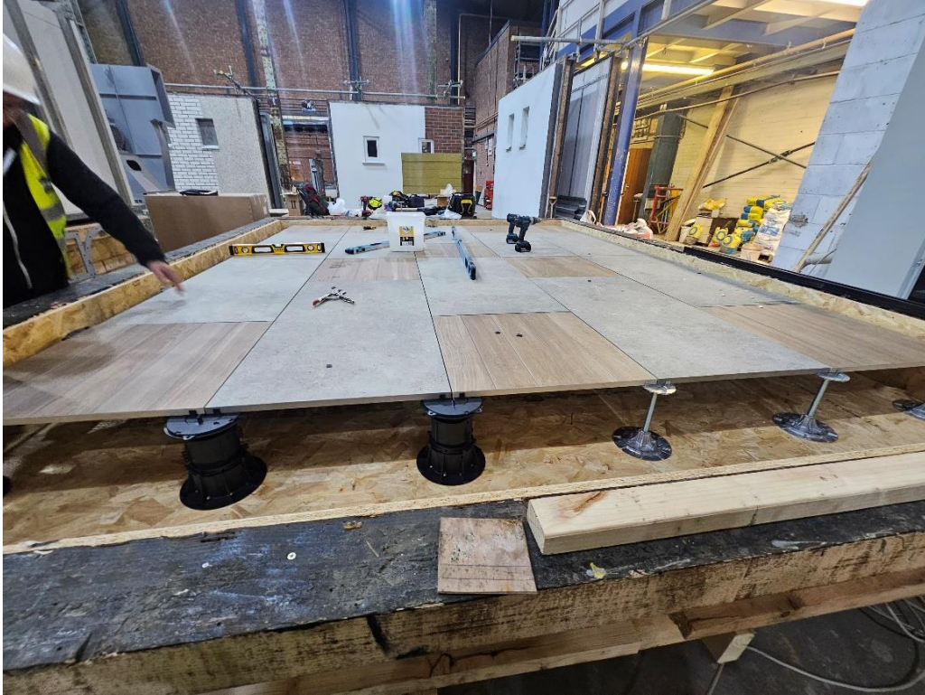
Plate 5 – Buzon A-PED and Buzon DPH Pedestals with Tiles
