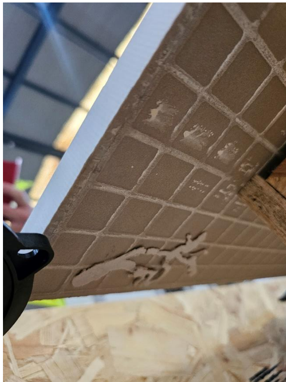
Plate 22 – Typical Failure Beneath the Tile (debonding of the adhesive from the pedestal)
