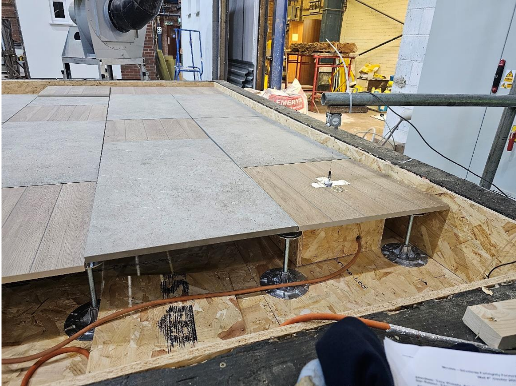
Plate 19 – Tiles Lifting During Load Testing
